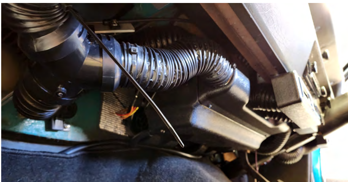
Photo 6 - Connect ducting & 32-16A adaptors to 32-18AX Y piece
