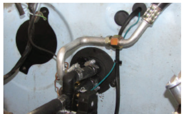
Photo 15 - Evaporator Outlet Tube
